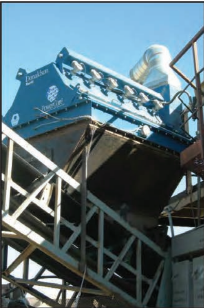
CPV-12 Conveyor line at concrete and asphalt plant 8,160 m 3 /Hr
