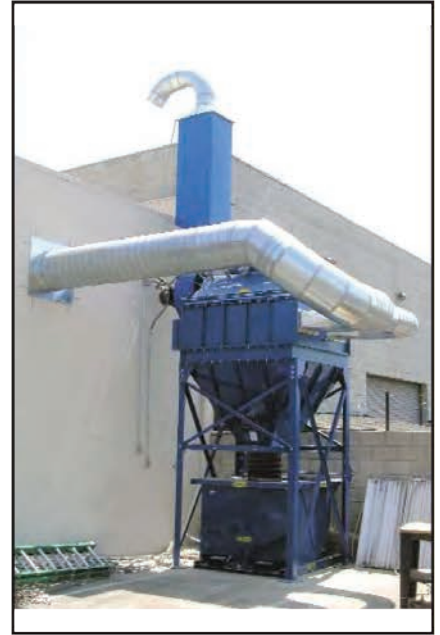
CPC-12 on wood dust at furniture manufacturer 11,900 m 3 /Hr
