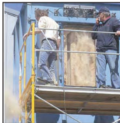
Bridged and packed baghouse.
