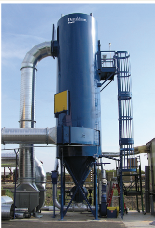
RF DUST COLLECTOR
